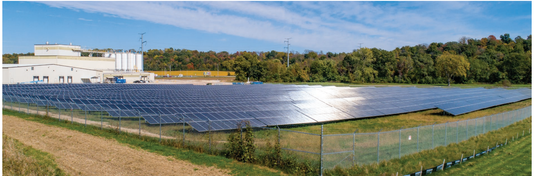
The solar array system at the HAM site in Marblehead, Illinois.
